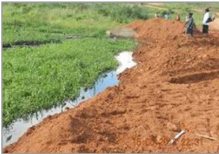
Construction of roads in wetlands limits flow of water.
